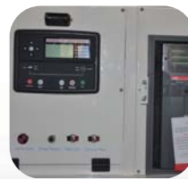
Control Panel & MCB
